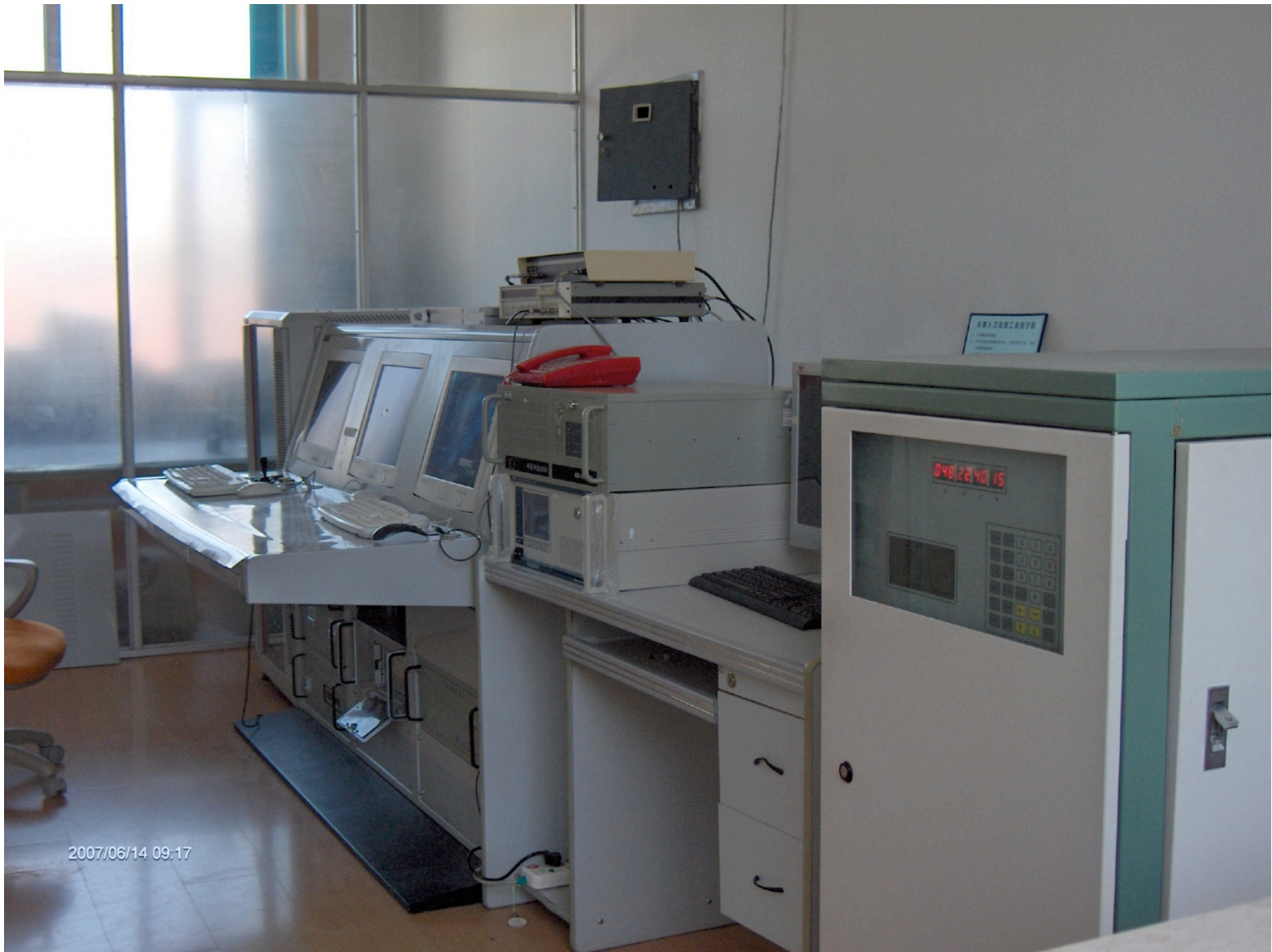
Changchun SLR Control Room
